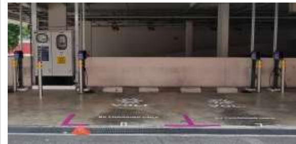
Electric vehicle charging points at the Woodlands Central Cluster
